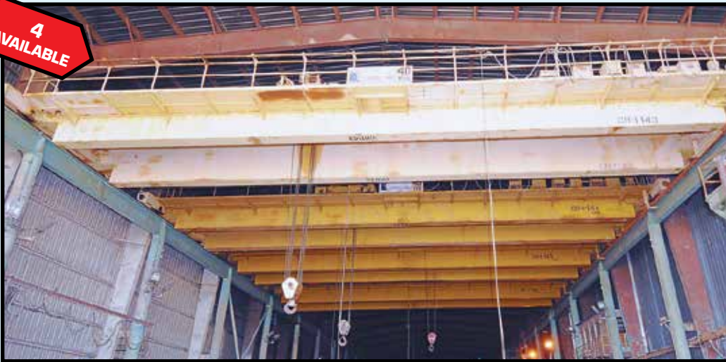
LANDEL 40 T. OVERHEAD BRIDGE CRANES
