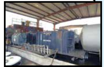
OIL STORAGE AND RECOVERY FACILITY
