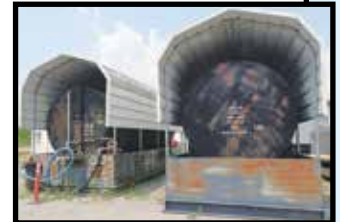
OILY WATER STORAGE TANKS
