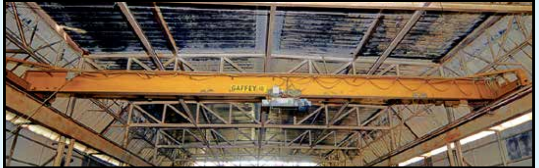
GAFFEY 10 T. SGL. GIRDER OVERHEAD BRIDGE CRANE
