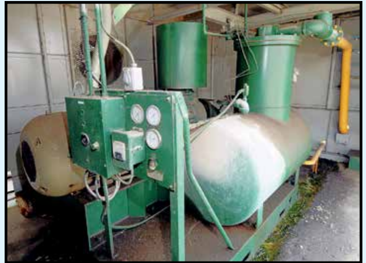
SULLAIR 300 HP ROTARY SCREW AIR COMPRESSOR
