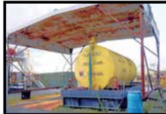
7,000 GAL. DIESEL STORAGE TANK STATION
