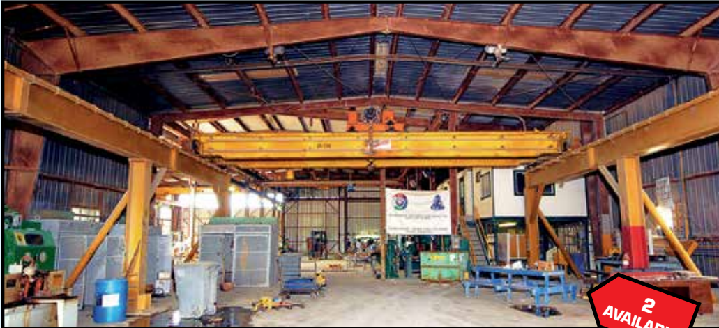
KRANCO 25 T. BRIDGE CRANES ON FREE-STANDING RUNWAY
