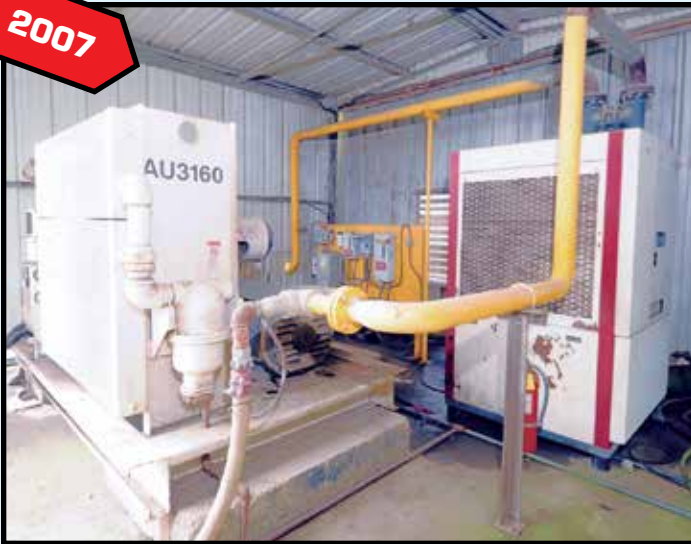
GARDNER DENVER 300 HP COMPRESSOR AND DRYER
