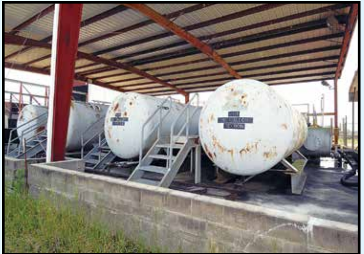
OIL STORAGE AND RECOVERY FACILITY
