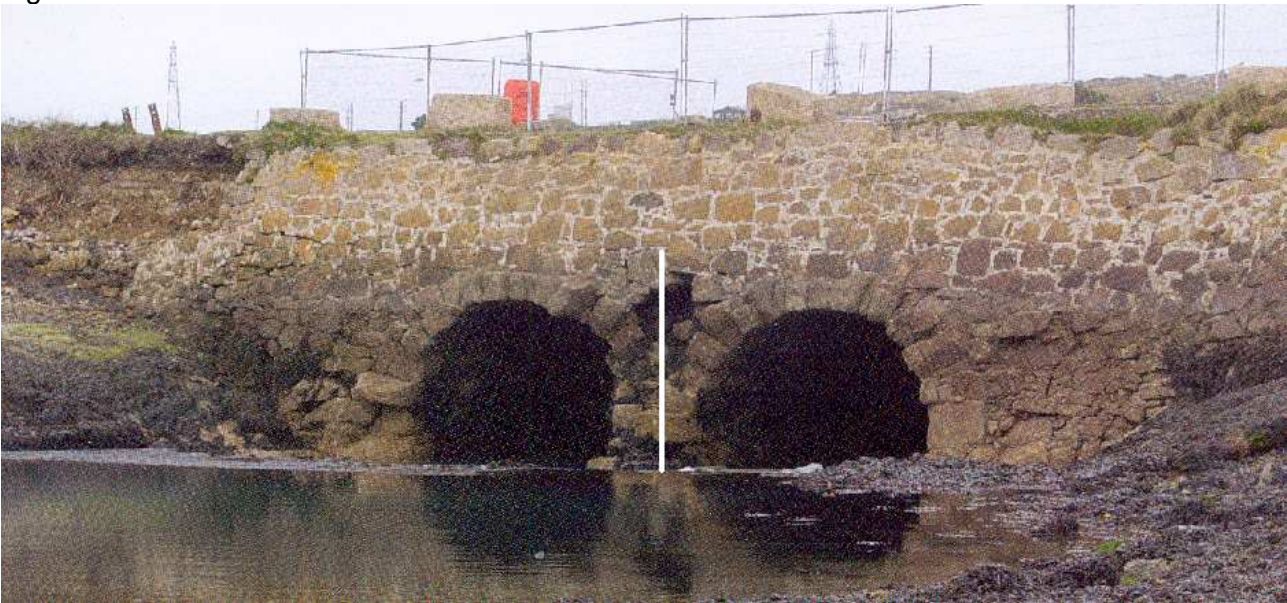
Figure 5: Sluice gate tunnels and weir photographed from within Carnsew Pool. The white line represents the height between the weir and the MHW level.
