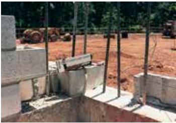
Doweling rebar into concrete foundation wall prior to building concrete block wall using G5.
