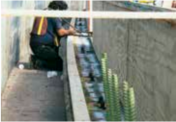
Doweling rebar into bridge deck and forming to pour new barrier wall using G5.
