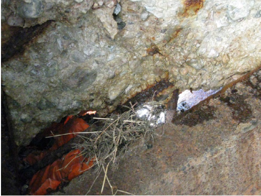
Photo 40: Bridge N-21-F – Exposed Rebar and Hole Through Deck Source: CDOT
