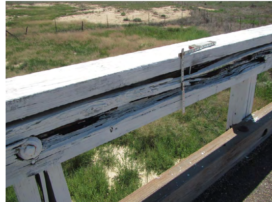
Photo 29: Bridge M-21-J – Heavy Splintering of Guardrail Source: CDOT
