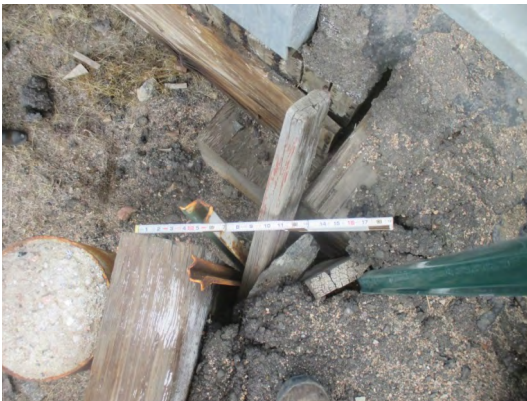
Photo 5: Bridge J-14-C – Wing Wall Displaced 13 Inches Source: CDOT
