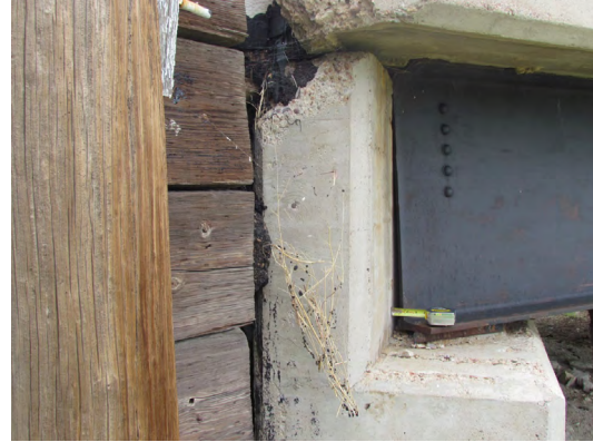
Photo 41: Bridge N-21-F – Displacement and Twisting of Girder due to Abutment Rotation Source: CDOT
