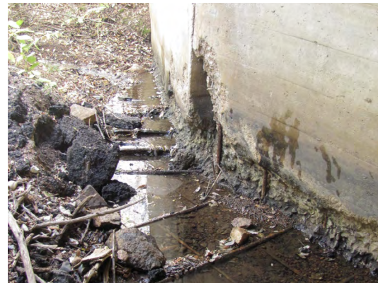
Photo 17: Bridge I-15-T – Exposed Bottom Slab Rebar at Wall Interface Source: CDOT
