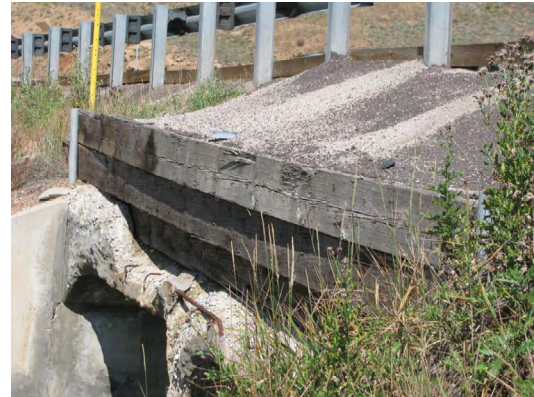
Photo 14: Bridge I-15-AO – Disintegration of Concrete Source: Google, CDOT
