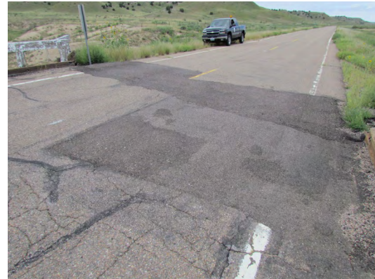
Photo 38: Bridge N-21-C – Wearing Surface Deterioration Source: CDOT
