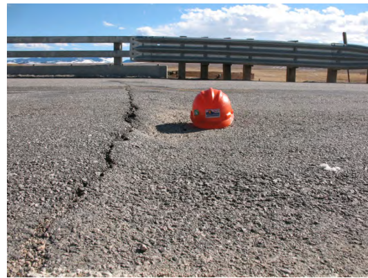
Photo 20: Bridge H-13-N – Settling of Roadway Source: CDOT
