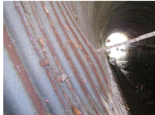
Photo 9: Bridge J-15-G – Bulging of Pipe Source: CDOT
