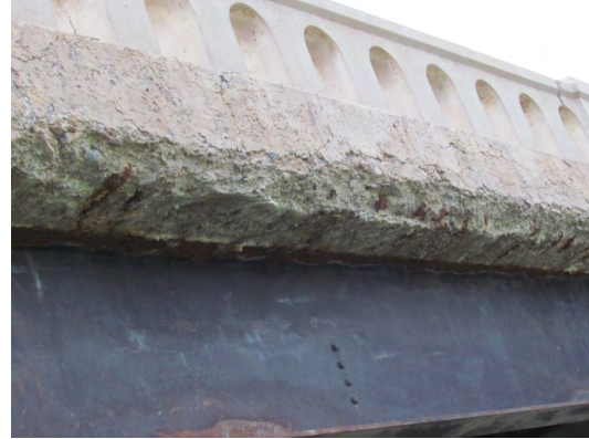
Photo 23: Bridge M-21-B – Typical Deterioration of Deck Overhang Source: CDOT
