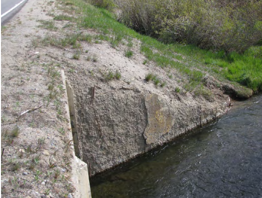
Photo 2: Bridge G-12-C – Disintegration of East Wing Wall Source: CDOT
