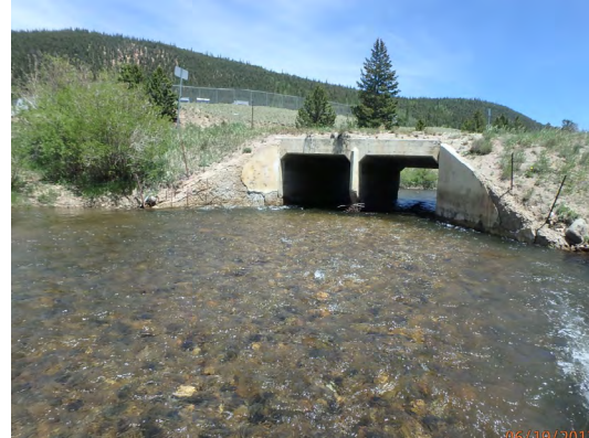
Photo 3: Bridge G-12-C – Disintegration of West Wing Walls Source: CDOT
