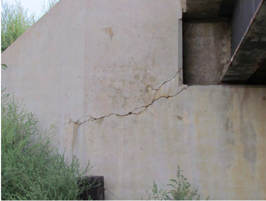
Photo 22: Bridge M-21-B – Typical Cracking of Substructure Units Source: CDOT
