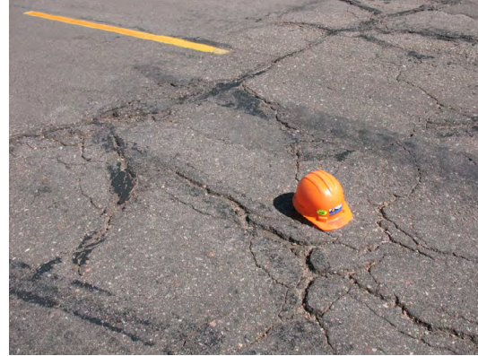
Photo 32: Bridge M-22-U – Deteriorated Wearing Surface on Approach Source: CDOT
