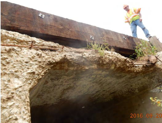
Photo 16: Bridge I-15-T – Deteriorating Concrete and Timber Retaining Wall Repair Source: CDOT
