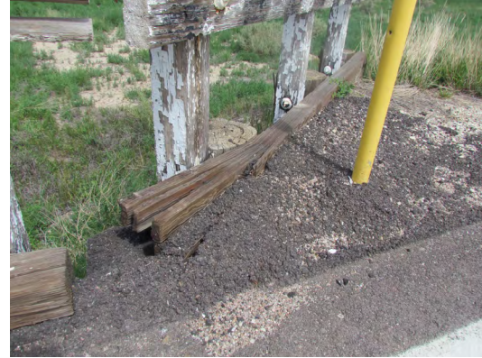
Photo 35: Bridge M-22- Y – Splintered Wing Wall Source: CDOT
