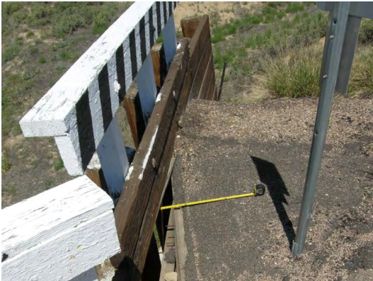
Photo 37: Bridge N-21-C – Displaced Wing Wall Source: CDOT
