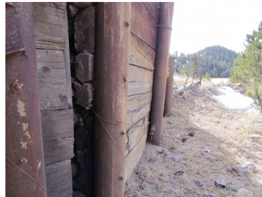
Photo 6: Bridge J-14-C – Bulge in Wing Wall Source: Google, CDOT
