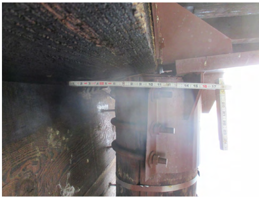
Photo 19: Bridge H-13-N – Deflection of Repaired Piling Source: CDOT
