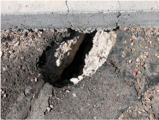
Photo 25: Bridge M-21-C – Hole in Deck at Pier Joint Source: CDOT
