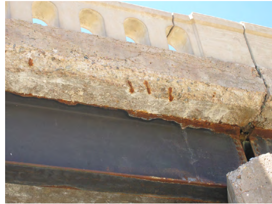
Photo 26: Bridge M-21-C – Deterioration of Concrete and Exposed Rebar Source: CDOT
