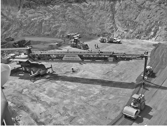
FIGURE 20.1 Placing RCC with 110 lb of cement and 54 lb of fly ash per cubic yard using a 24-in. conveyor at Rompepicos Dam, Mexico. (Photograph courtesy of Ernest K. Schrader.)
