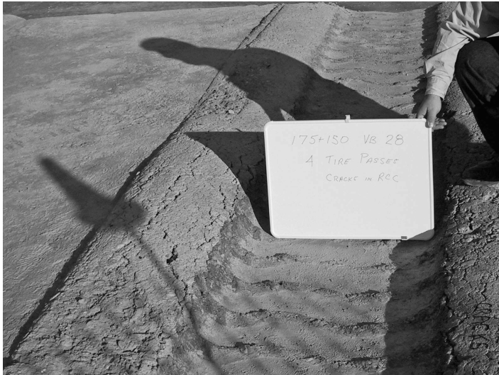
FIGURE 20.16 Surface damage caused by truck tires on wet-mix RCC.
