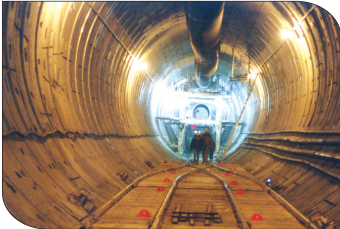
Figure 23. St. Clair river tunnel precast tunnel lining segments. (Courtesy Hatch Mott MacDonald)
