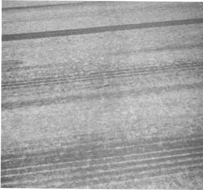
Photo 1. Transverse crack in reinforced PCC slab of NW-SE runway
