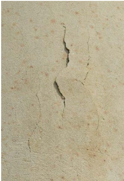
Figure 3. A detachment on the shaft of column L20, which is has not progressed to contour loss.
