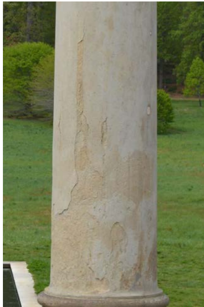
Figure 4. The lower shaft of column L20 has the highest contour loss, extending more than six feet; a detached area reaches even higher. The area of detachment can be seen on the left.
