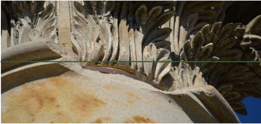
Figure 7: Detail of stone loss from L13's astragal, revealing its iron ring directly below the bottom edge of the capital.
