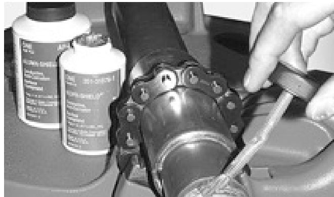
Figure 20: Application of UL listed electrically conductive occasion protection compound on field-cut threads.
