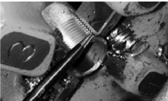
Figure 9: When proper thread length is achieved the end of the conduit becomes flush with the ends of the die segments.
