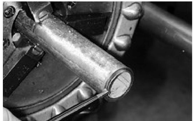
Figure 6: The roll cutter will leave a burr on the inside diameter of the conduit. The burr must be removed to ensure that the wire insulation will not be damaged during pulling.
