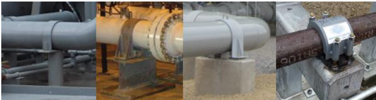
Figure 11. Example of various piping support structures with clamp-type restraints
