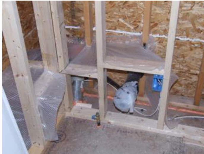
Figure 9. Insulation netting surrounds vents and plumbing penetrations in an exterior double wall.
