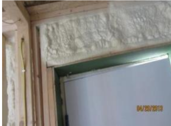
Figure 12. Reductions in framing around the openings allows for more insulation in headers.
