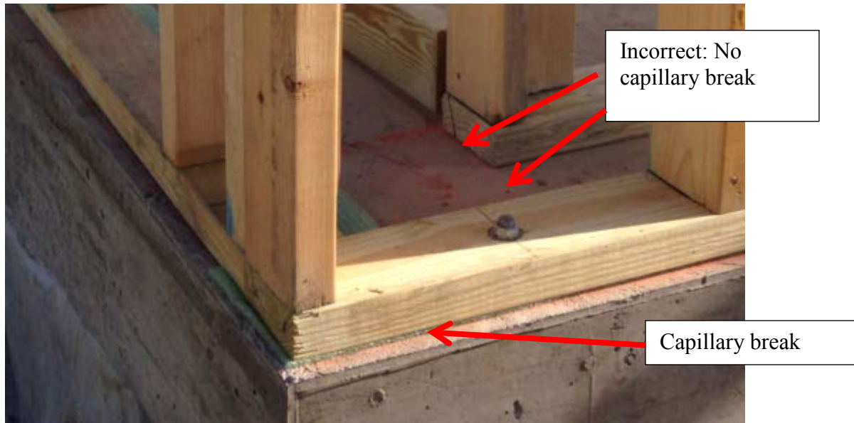
Figure 17. Incomplete capillary break. It should be installed the entire depth of the wall to keep lumber and insulation from wicking up moisture.
