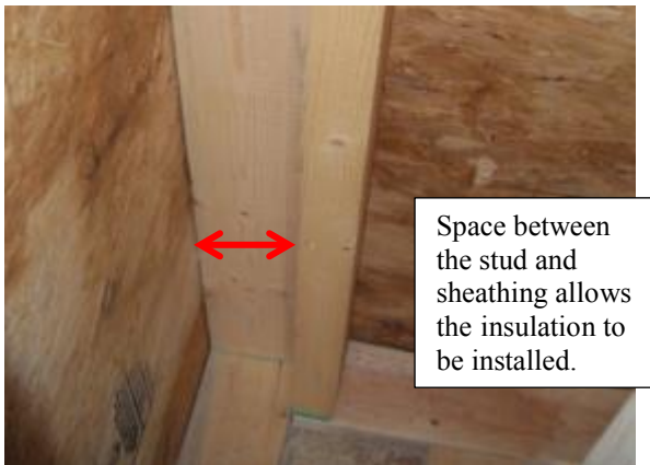
Figure 10. Two-stud corners can be used for both the interior and exterior walls in the double-wall assembly.
