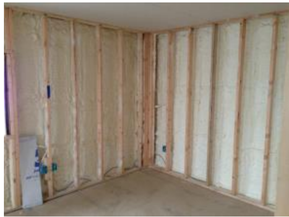
Figure 3. ccSPF in the outer stud cavity of a 12-in. double wall. Cellulose will fill the remainder of the cavity.
