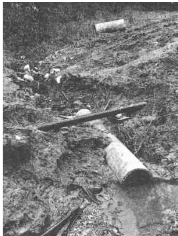
Figure 3. Drainage line which has not been stabilized early.
