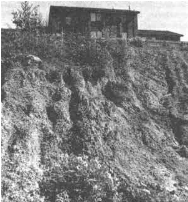
Figure 1. Eroded embankment and driveway which have not been stabilized during early stages in a housing subdivision area
