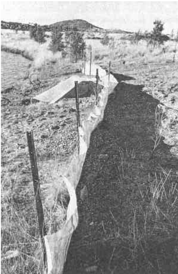
Figure 34. Filter cloth sediment trap fence used to trap sediment from a small catchment.
