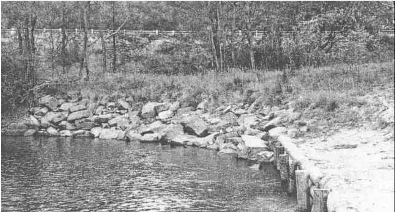
Figure 18. Steep river bank stabilised by a thick layer of rock near a roadway.
