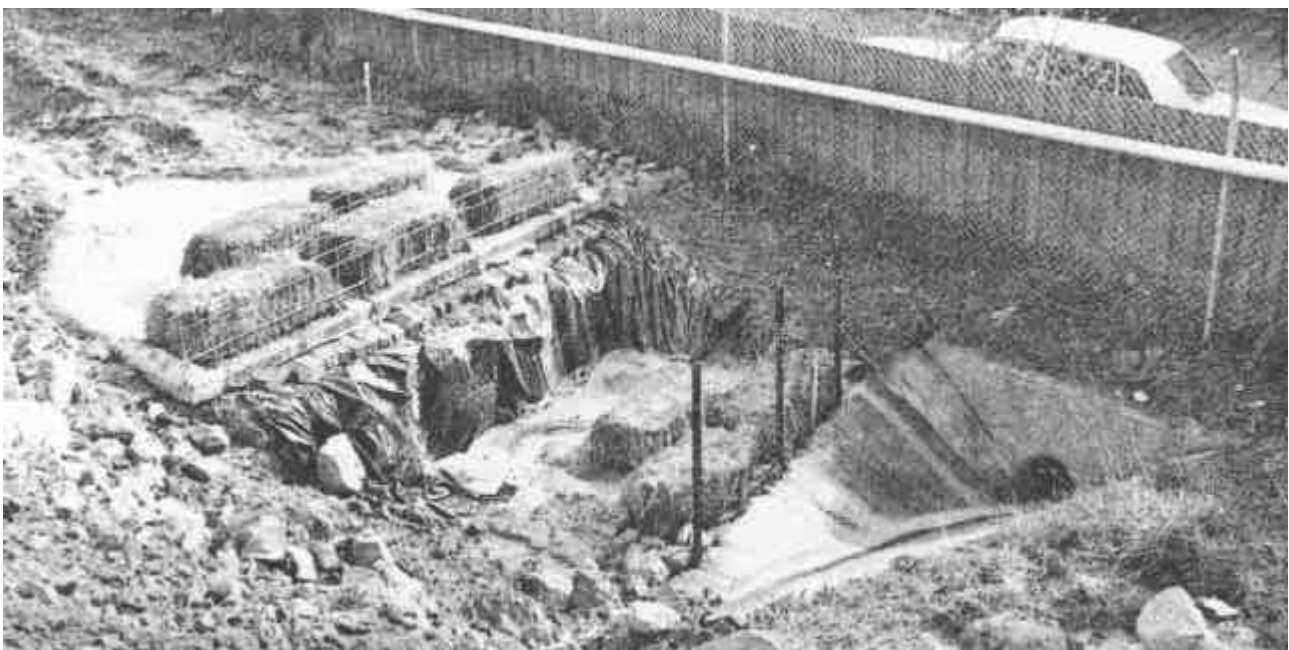
Figure 30 Sediment trap featuring litter screens to prevent pipe blockage and concrete and plastic aprons to prevent undercutting.
