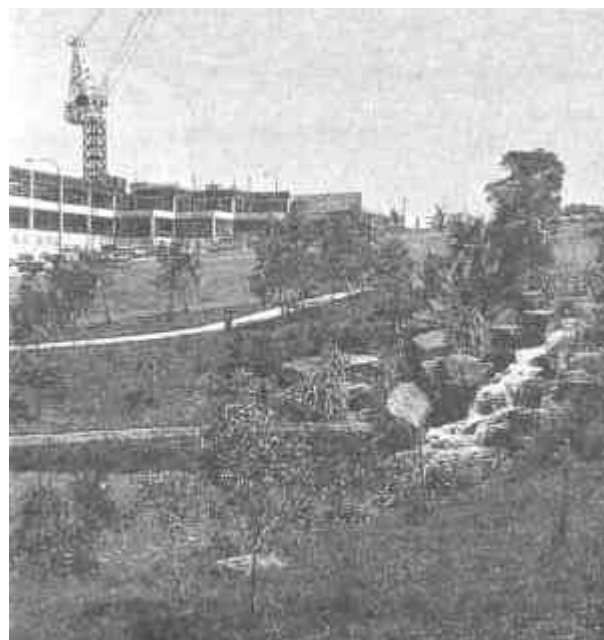
Figure 4. Drainage line and hillside which have been stabilized during early construction stages.
