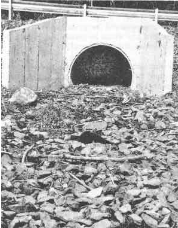
Figure 25. Pipe outlet protected from erosion by a thick layer of rocks.
