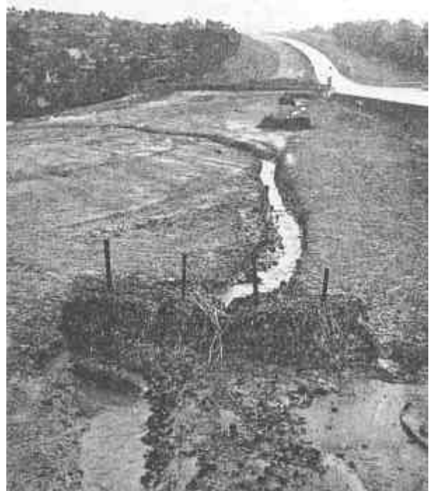
Figure 31. This hay bale sediment trap has not been effective because the channel is steep and unstabilized. This has resulted in erosion along the channel and around the sides of the bales.
