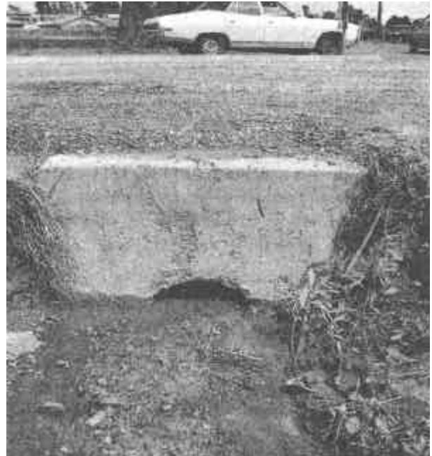
Figure 2. This sediment from a roadside drain blocks stormwater pipes and can pollute rivers and creeks further downstream.
