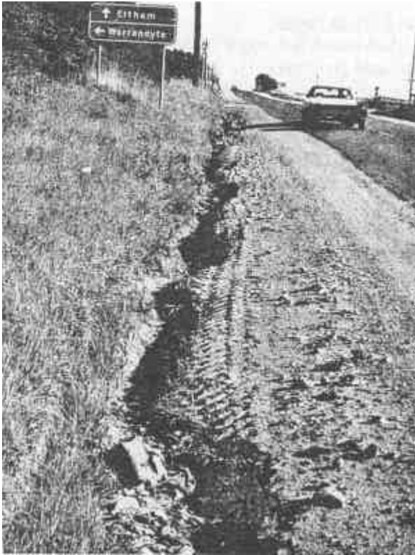
Figure 39. Eroded roadside table drain which contributes to sediment pollution.
