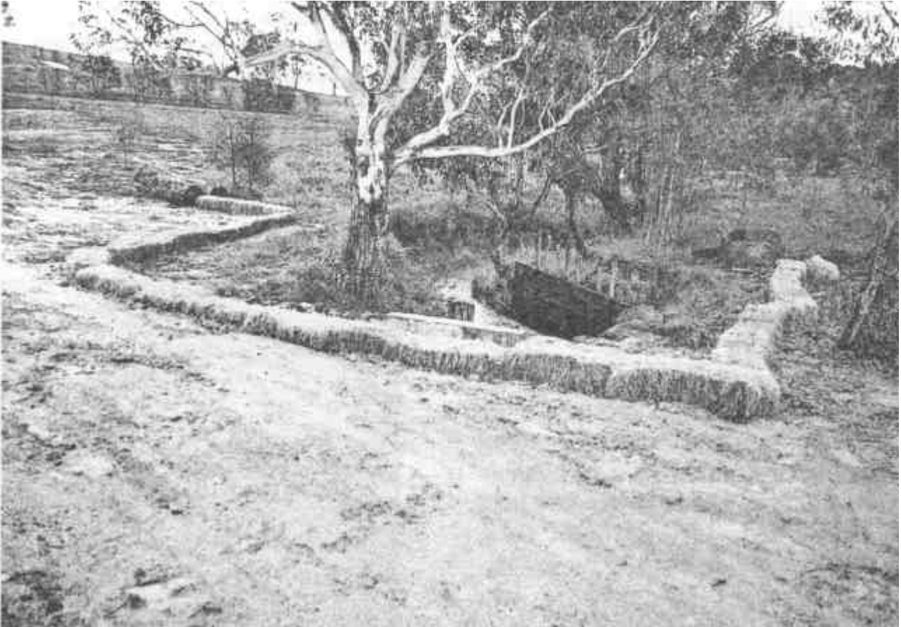
Figure 33. Row of entrenched hay bales which traps sediment and diverts muddy water into densely grassed areas.
