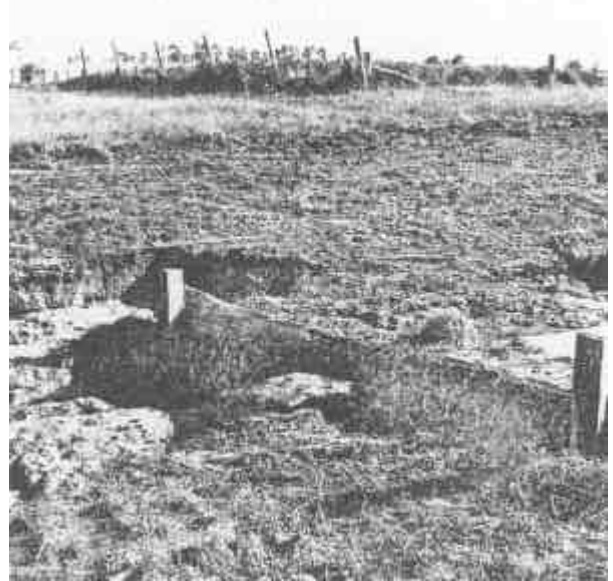
Figure 22. Poorly designed structure which has been undermined and side scoured
