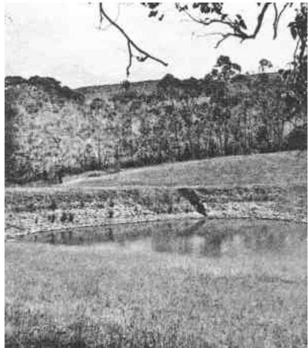
Figure 28. Dam embankment which has been breached by water as a result of poor soil compaction.
