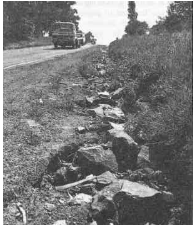
Figure 16. A few large rocks by themselves are seldom adequate to prevent side scour.
