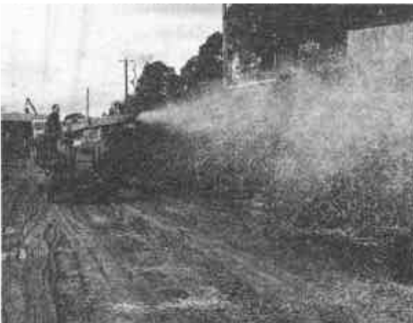
Figure 8. Chopped straw and bitumen being blown onto a batter. Care is needed to prevent bitumen drifting onto nearby property.
