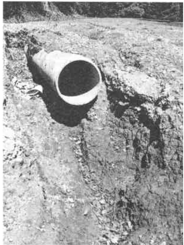
Figure 24 Soil erosion has undermined this pipe outlet and contributes to sediment pollution.
