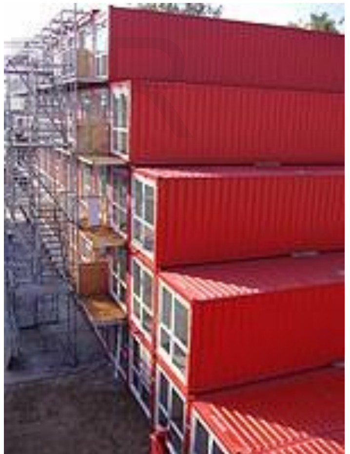
Fig 29: using a distinctive color helped in creating an eye-catching mass of rooms.
