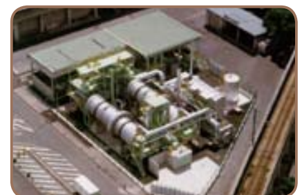
Kitchen garbage volume reduction plant
