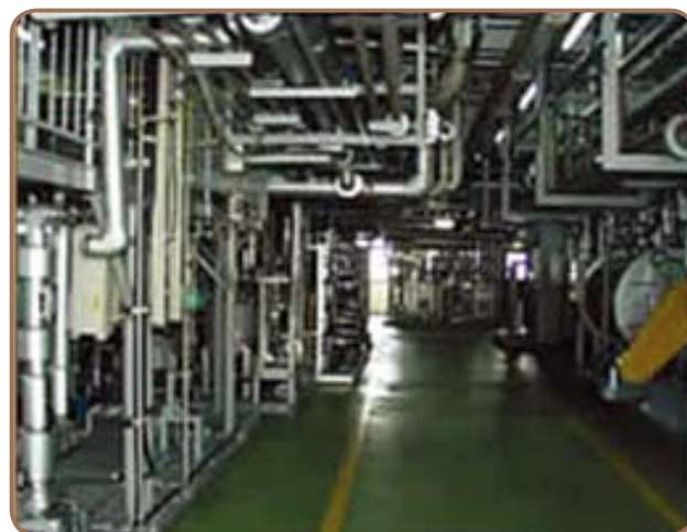
Separation and crystallization facilities
