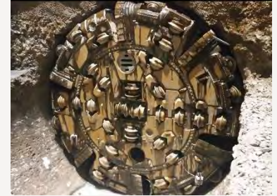
Indianapolis, IN / Deep Rock Tunnel Connector, Phase 1: 8 miles, 20 ft. diam. ww tunnel - $179M
