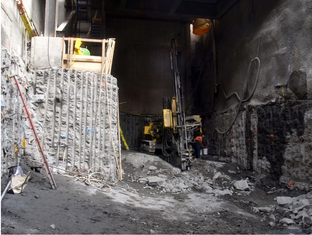
Figure 7 – Northward view of ancillary cavern of Second Avenue Subway 86 th Street Station complex showing line drilling in progress in excavation floor and line-drilled walls. This sensitive excavation (adjacent buildings) went down nearly 100' more by April 2013 by stepping downward in lift increments. (C. Merguerian digital image taken 06 November 2012.)
