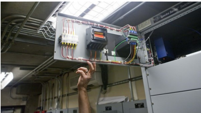
The Utilities unit provides whole-building energy monitors to document the savings generated when fume hoods are lowered. This is a smart electricity meter. All of the other meters connect into this meter for communication with our central databases.
