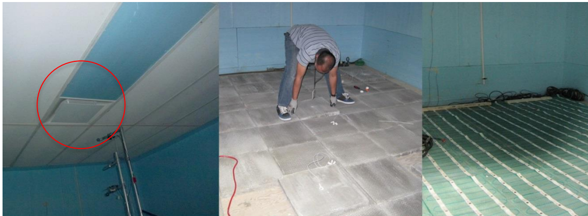
Radiant panel and air diffuser setup
