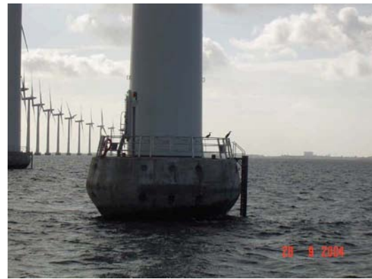
Figure 9: The access ladders for smaller boats are damaged after winters with ice. A special weak link is build into the ladder in order to limit the damage.
