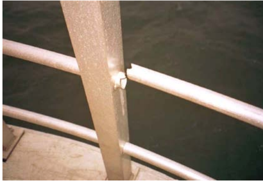
Figure 8: The distance between the posts in the fence has been too large creating vibrations caused by the wind. The repair is simple.
