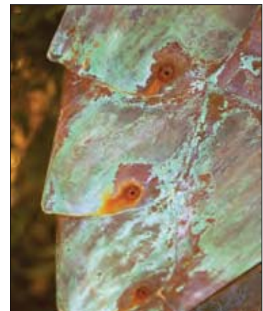
Figure III-10. Steel rivets used to join sections of exposed copper sheet create an ideal opportunity for galvanic corrosion. In this case, less noble steel corrodes while more noble copper remains protected. Corrosion is accelerated by large differences in area size between the two metals.
