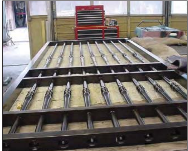
Figure VI-12. Oil-rubbed bronze gates prepared for installation at the State Capital in Harrisburg, Pennsylvania.
