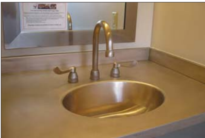
Figure I-3. Antimicrobial Copper sink and faucet installed at the Ronald McDonald House of Charleston, South Carolina. Healthcare facilities around the world are recognizing products made from EPA-registered Antimicrobial Copper alloys continuously kill bacteria that cause infections. The sink is made by Elkay Commercial Products and the faucet by Rocky Mountain Hardware.
