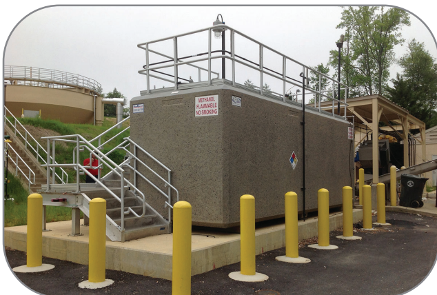
Waste Water Treatment Plant in Maryland
