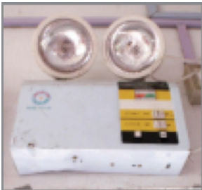
Example of emergency lighting.
