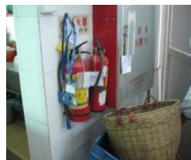
Example of blocking of fire equipment.
