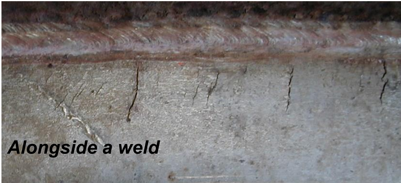
In the wall of a stainless steel pipe
