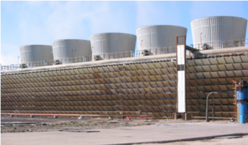
Figure 17. Corrosion in a cooling tower of a geothermal power plant.
