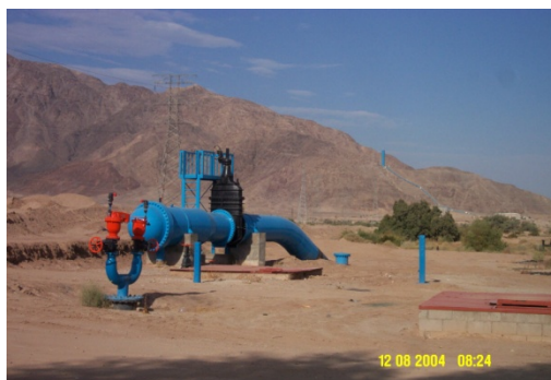
Figure 7. Valve system of a desert water aqueduct.
