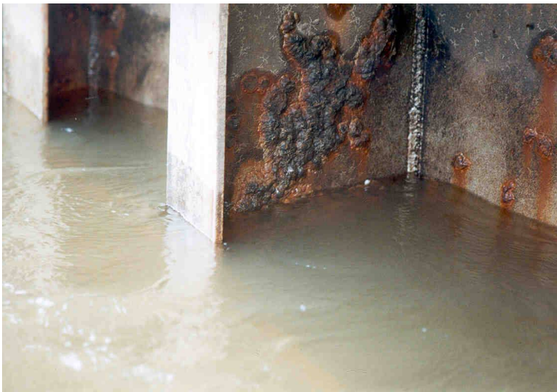
Figure 5. Corrosion on the gates dam on the Colorado River, Baja California, Mexico
