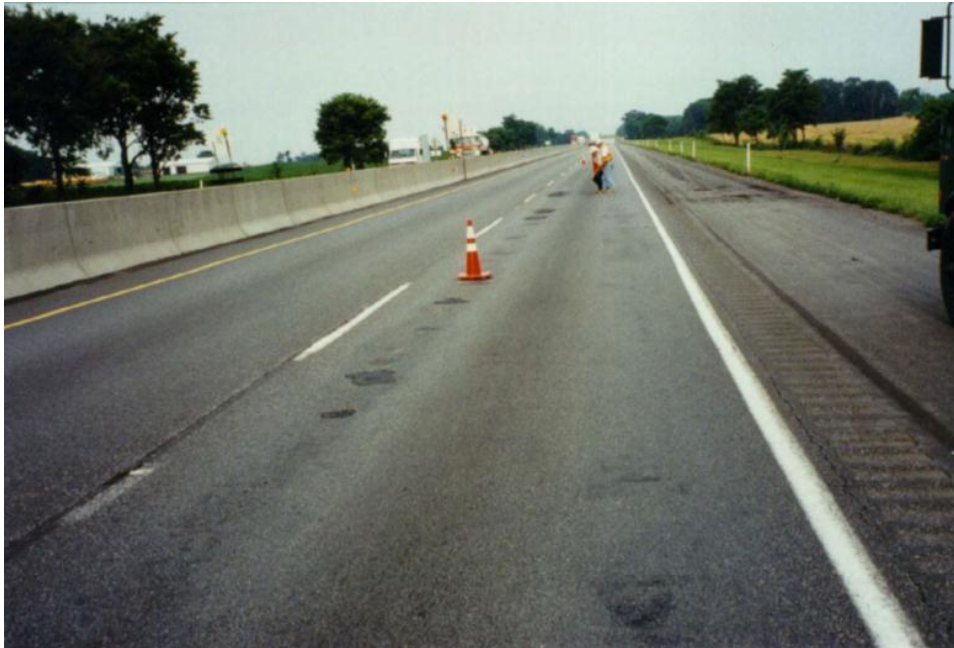
Figure 8. Pennsylvania Turnpike Westbound Lane Near Milepost 217.65, Showing Potholes Due to Moisture Damage (Kandhal and Richards, 2001).
