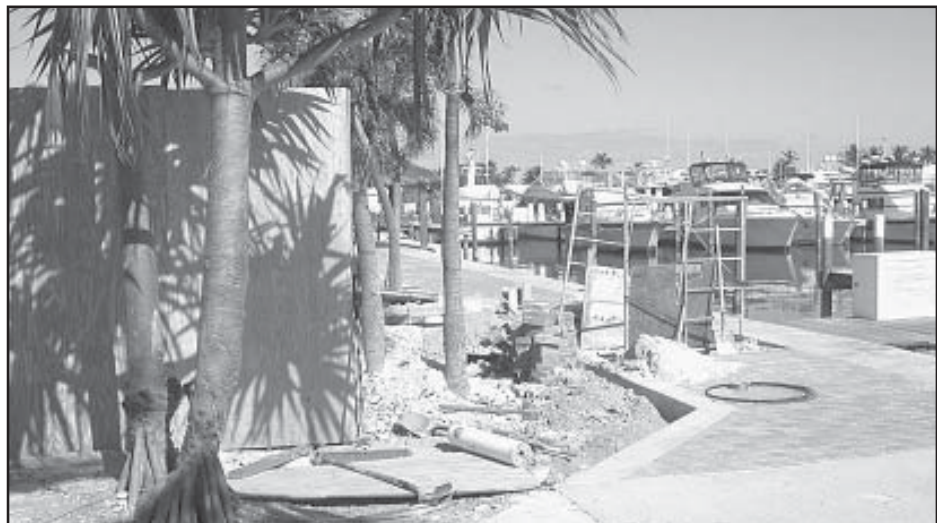
Construction is underway at the Abaco Beach Resort as it begins a major expansion program. The resort will eventually have a convention centre, additional restaurants and 100 condominiums. The resort hopes to encourage our visitors to spend more time here. Many business people also patronize the Abaco Beach Resort so it will cater to these business people as well as to visitors and second homeowners. "This large expansion will generate many jobs for Abaconians, not only during the construction phase, but on an ongoing basis for additional employees at the resort. It will have the positive effect of bringing more revenue into Abaco," stated Mr. Neophytou, resort manager.
