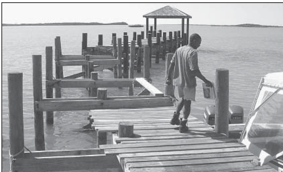
The government dock in Crown Haven is heavily used. The ferry to MacLean's Town on Grand Bahama uses it regularly as well as Little Abaco fishermen. However, it was badly damaged by the two hurricanes of 2004 and has not been repaired. It is dangerous to use but is the only dock available. Min. Bradley Roberts has said recently that someone is to come to repair all government docks in North Abaco.
