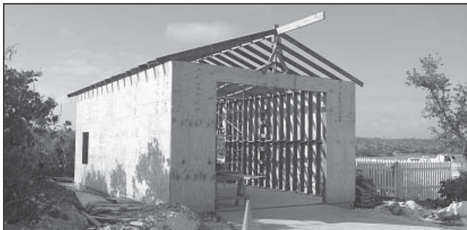
Construction work continues on Hope Town Volunteer Fire and Rescue's newest fire station which is located adjacent to Sea Spray Resort and will service the southern end of the island. The 640-square-foot building will accommodate one pumper truck and have sufficient space for a workshop area and storage. The new fire station is being built largely by volunteers from local construction crews working on Saturdays. It is hoped that the building will be completed by the end of March.
