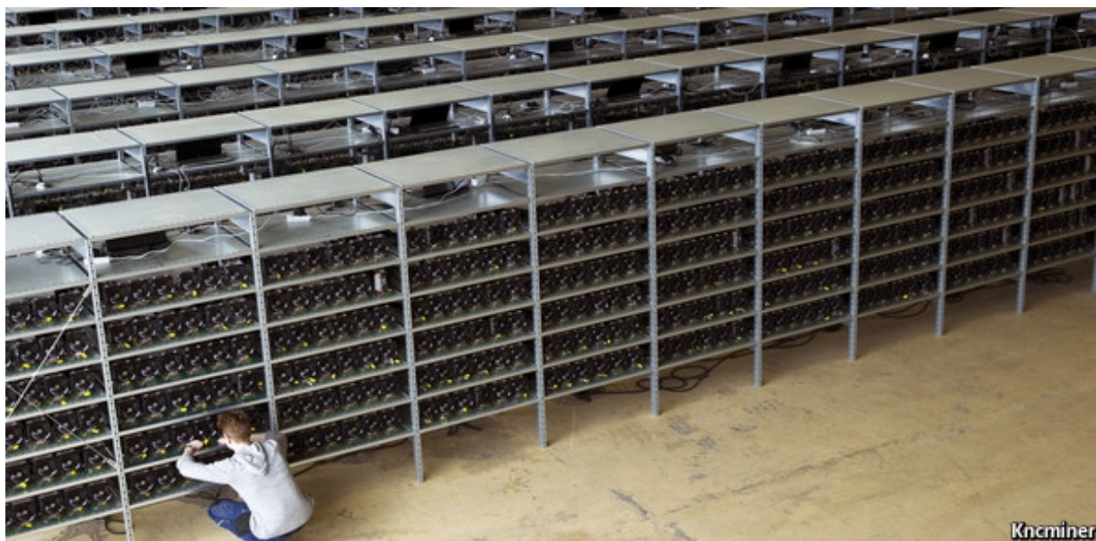
Image: Inside view of a Swedish mining farm 2 .
