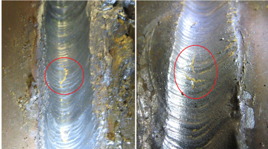
Figure 10 Magnetic particle tests to confirm presence of cracking
