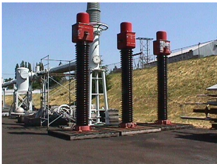
Oil filled 500kV
