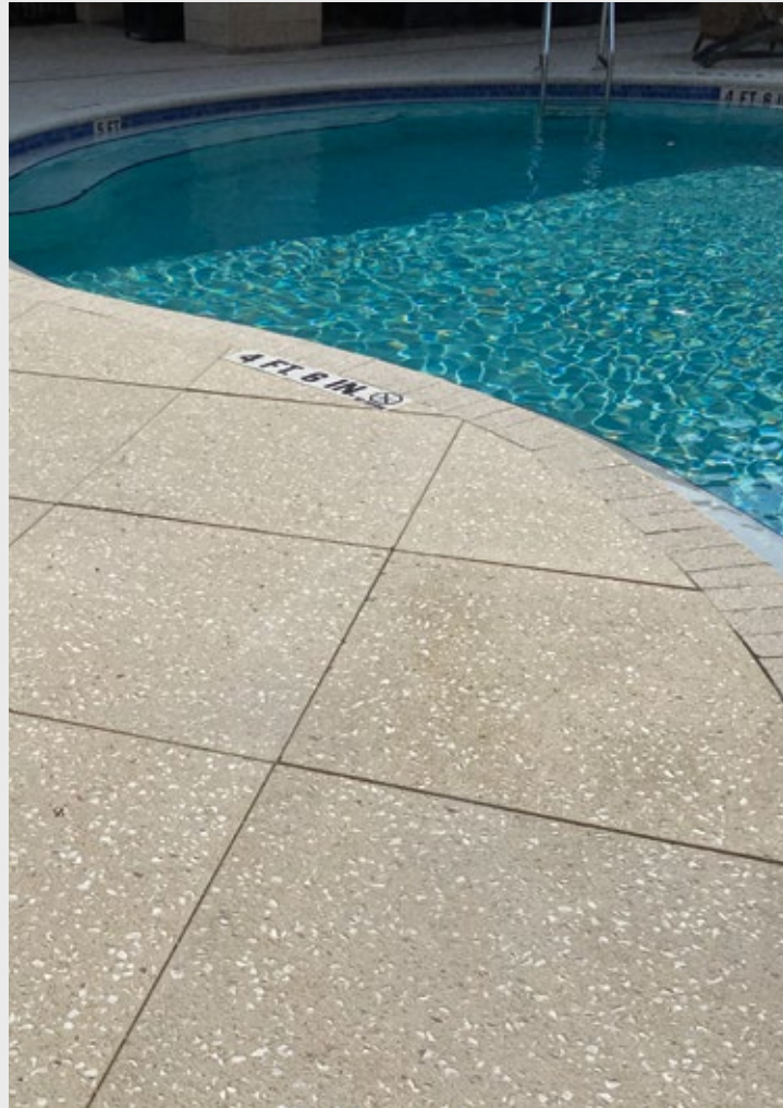
Brownwood Hotel & Spa | The Villages, FL | Custom Precast Concrete Pool Coping
