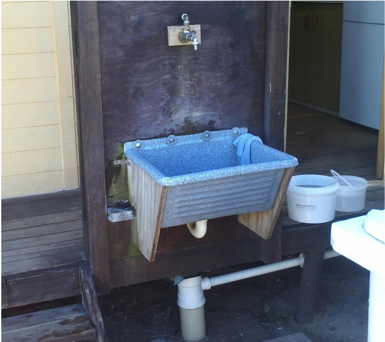
Figure 7 Drinking water tap at an NPO 30
