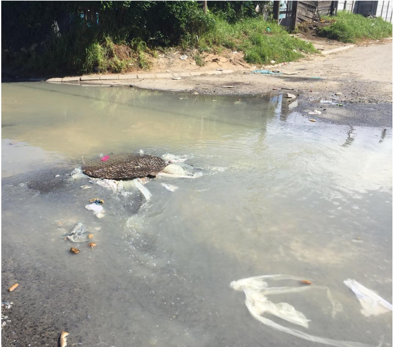
Figure 10 Overflowing manhole cover in Wallacedene 41
