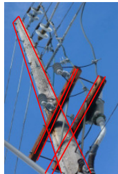
Poles and Crossarms
