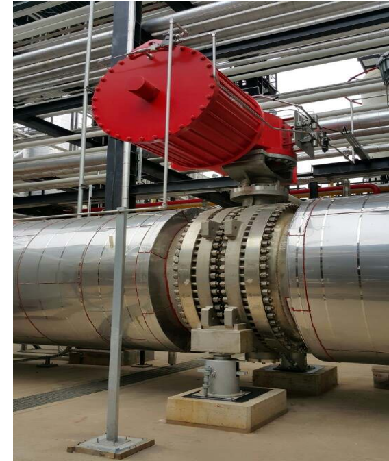
SK PDH PJT - 78inch Butterfly valve DESIGN TEMP. : 704°C OPERATING TEMP. : 625°C FLUID : REGENERATION GAS
