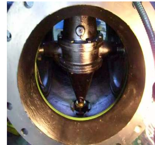
Operation of water seal valve.
