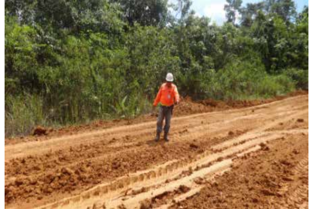
2. Grading of Village Road of Dirung Sararong RT I and RT II
