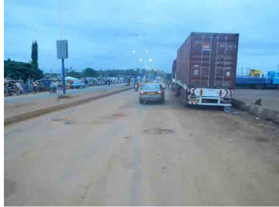
Road with pavement deterioration National Route 1 near the Sahel terminal, Togo
