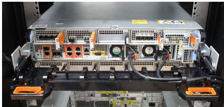
Figure 21 Cables organized on CMA
