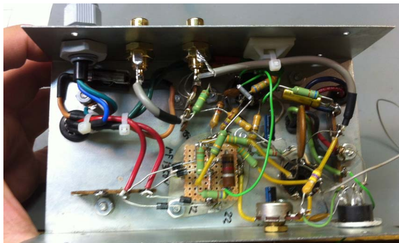
figure 31: wiring adapted to new transformer position
