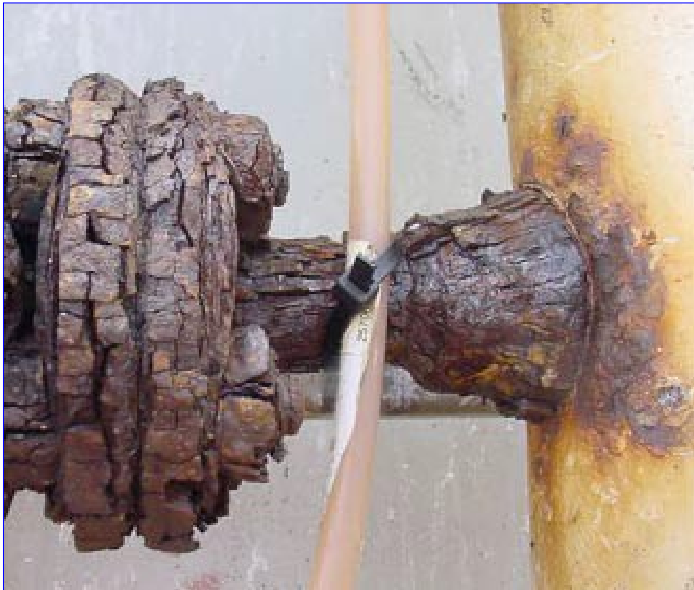
Lack of inspection and maintenance on a flange and bolts
