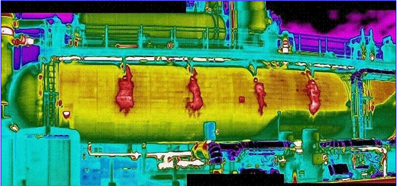
Thermal image of De-Salter vessel showing water intrusion under the insulation
