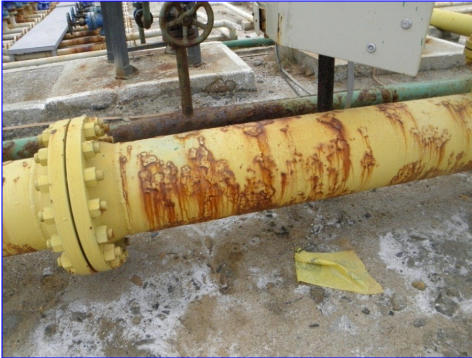
Paint breakdown and external corrosion
