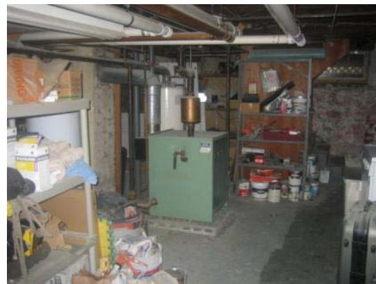
Steam boiler in basement
