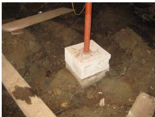
Standing water in basement
