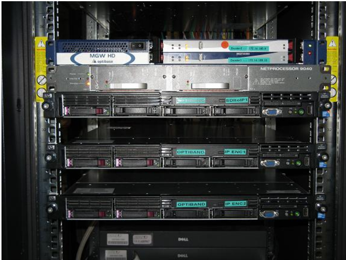
Figure 7: TVN and OPTEC Multi-rate Encoders in the System rack
