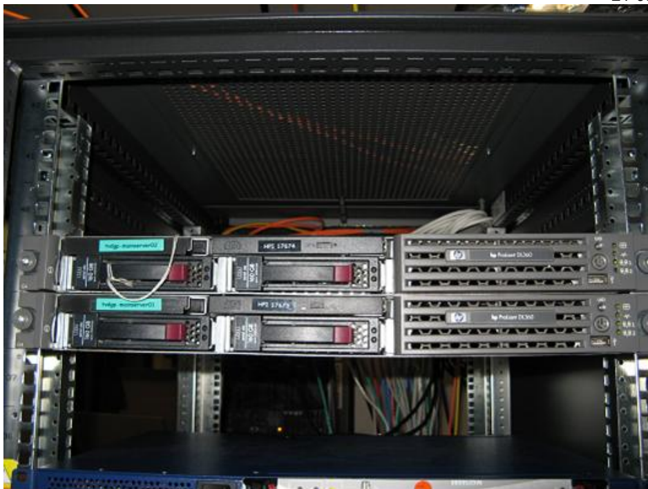
Figure 19: Installed servers for the SVC solution
