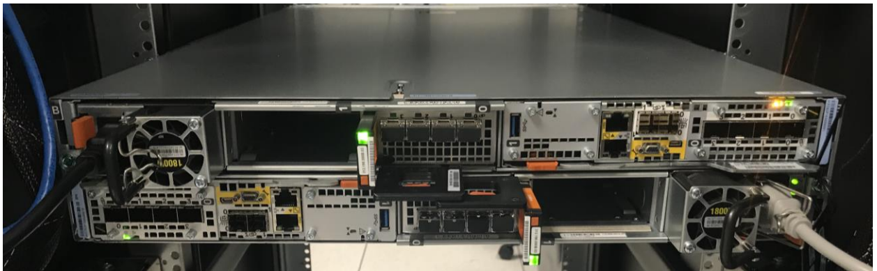
Figure 11. Rear of DPE (480/F, 680/F, 880/F)
