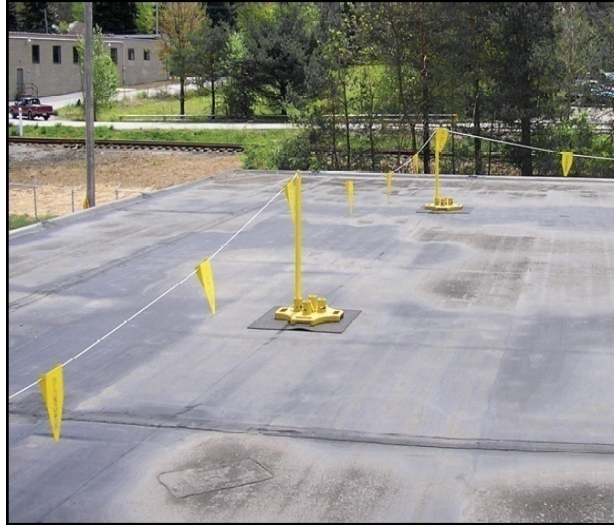
Warning Line System
