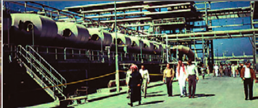
Figure 13. A single MSF unit at Al-Jubail Phase 2
