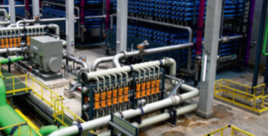
Figure 16. One example of energy recovery devices used in a SWRO plant
