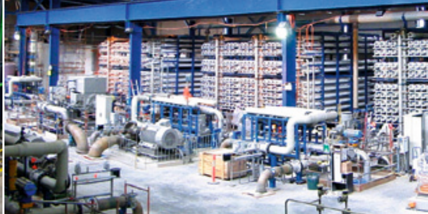
Figure 17. A typical large SWRO plant
