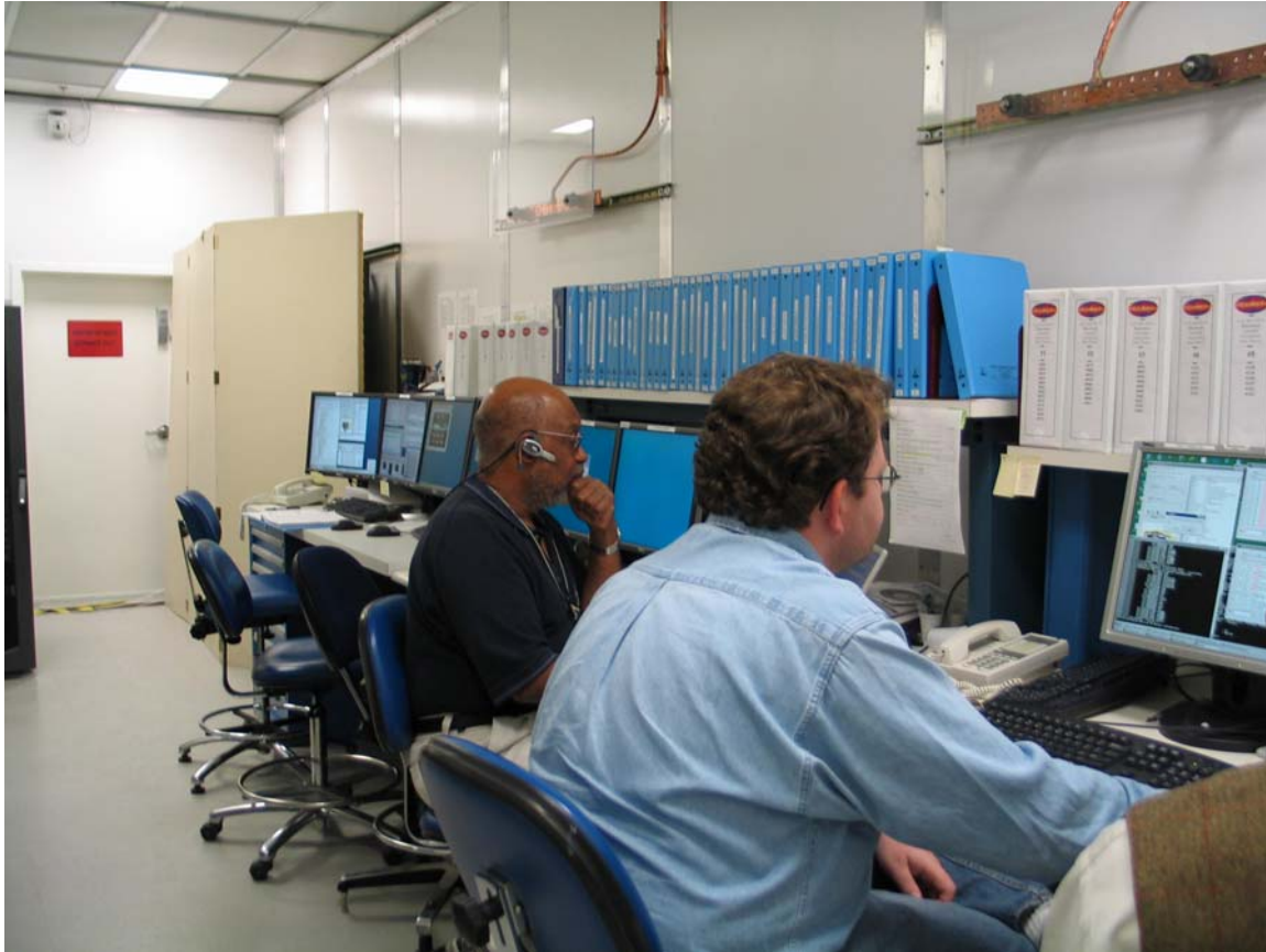
Figure 46: The LAT I&T facility control room (Room 102, Bldg. 33, SLAC)
