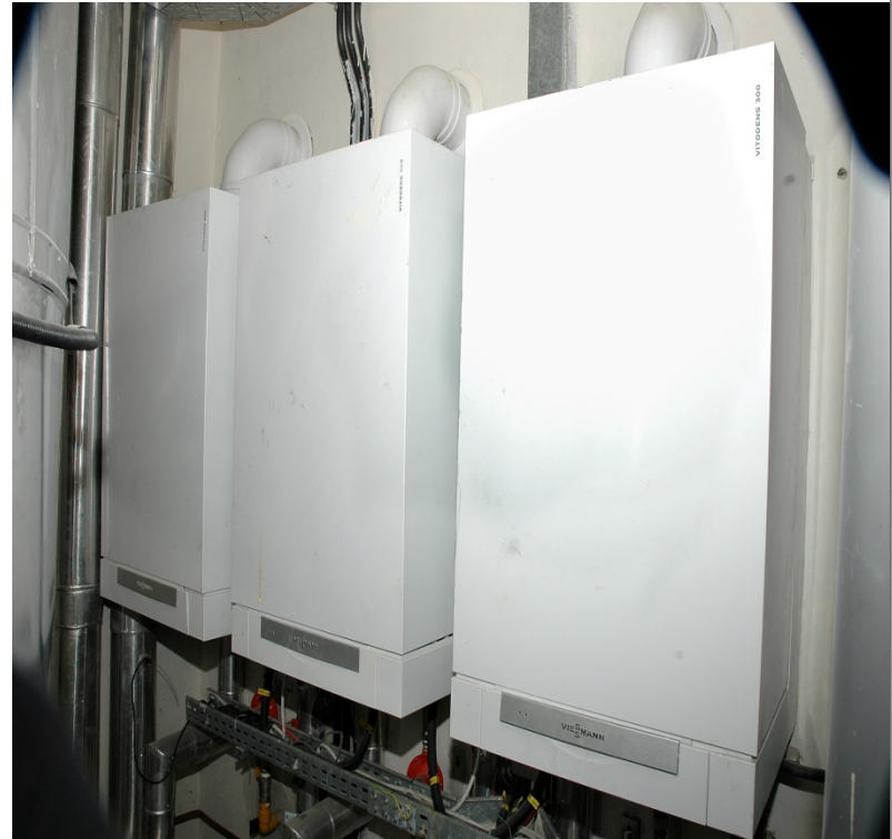
Viessmann Gas condensing boilers for the backup of the system (109 % efficiency)
