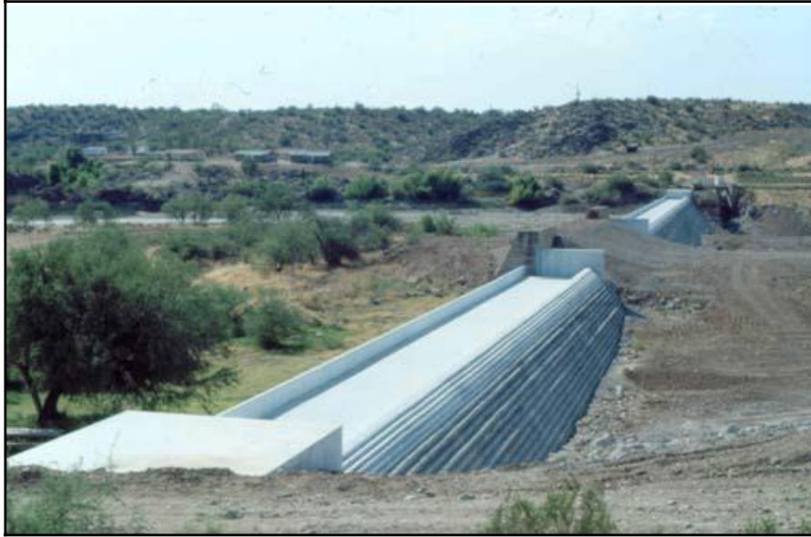
Figure 10-14. Completed Camp Dyer Diversion Dam and Dike, viewed from the right abutment (flow left to right).
