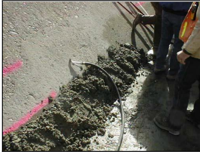
Figure 9-1. Leveling concrete used at Pueblo Dam at the interface between the existing concrete and the RCC. Note the surface preparation to develop bond between the existing and leveling concrete.
