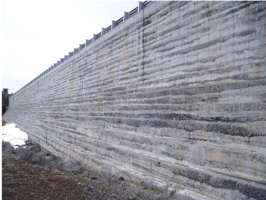
Figure 10-33. Photograph of the downstream face of Clear Lake Dam showing the formed RCC. Note the segregation that occurred against the forms during the RCC placements.
