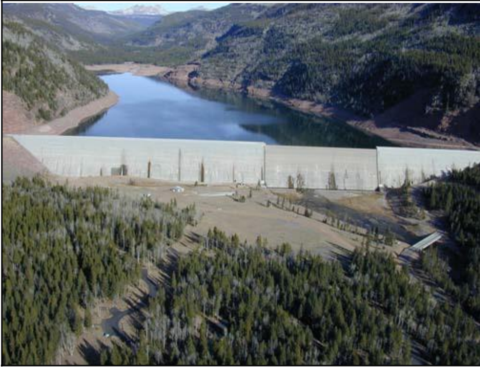
Figure 10-1. Aerial view of the completed Upper Stillwater Dam, showing the downstream face and seepage from cracks following the first winter and first filling.
