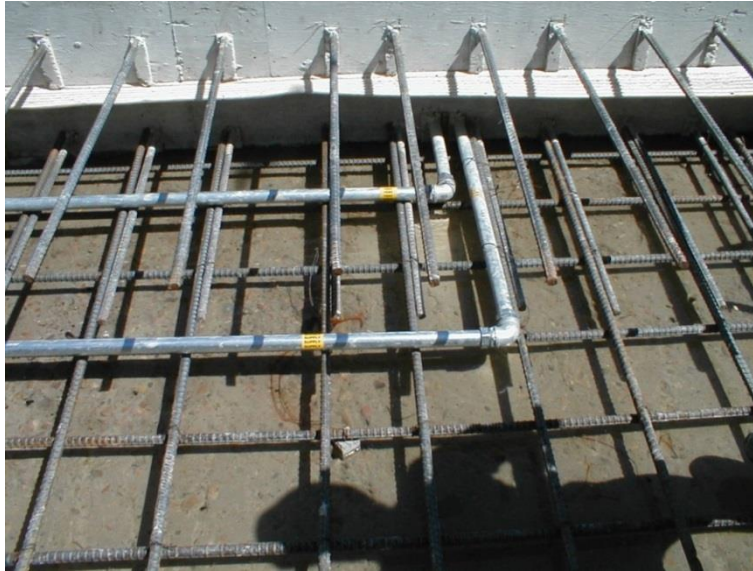
Figure 10-22. Conventional reinforced concrete overlay on the RCC placements. Note the embedded supply and return lines for RCC crack inducer joint grouting, as well as waterstops and reinforcement embedded in the conventional concrete overlay control joints.
