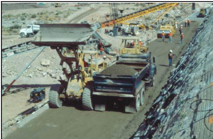
Figure 10-11. Heavy equipment safely passing on 20-foot-wide lift at Camp Dyer Diversion Dam.
