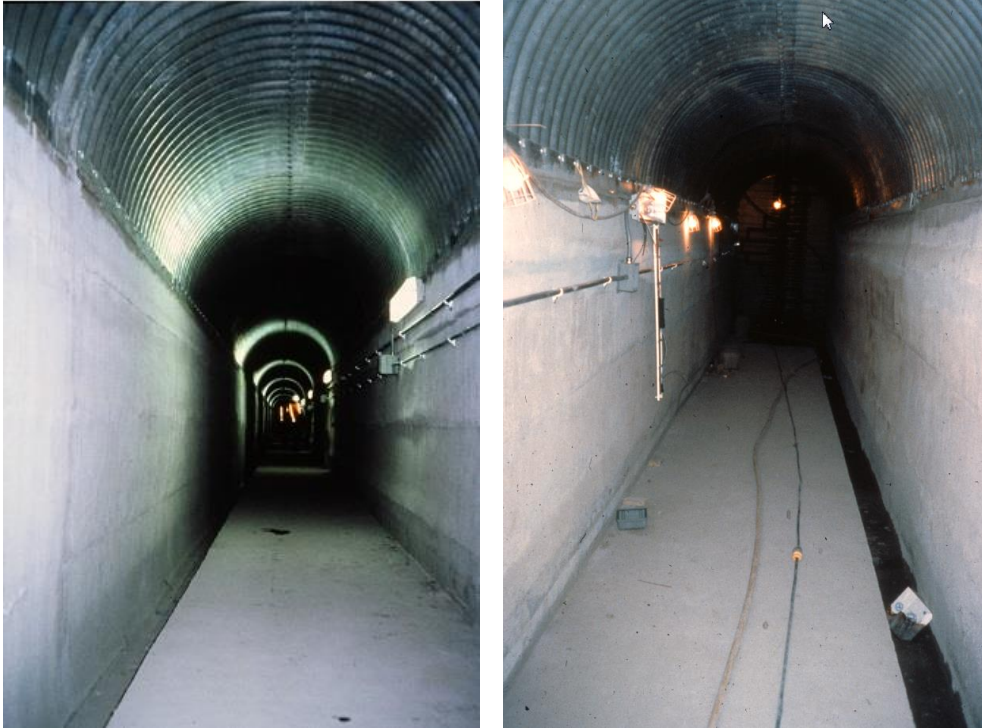
Figure 10-8. Gallery at Upper Stillwater Dam showing slipformed concrete walls and corrugated metal pipe crown.
