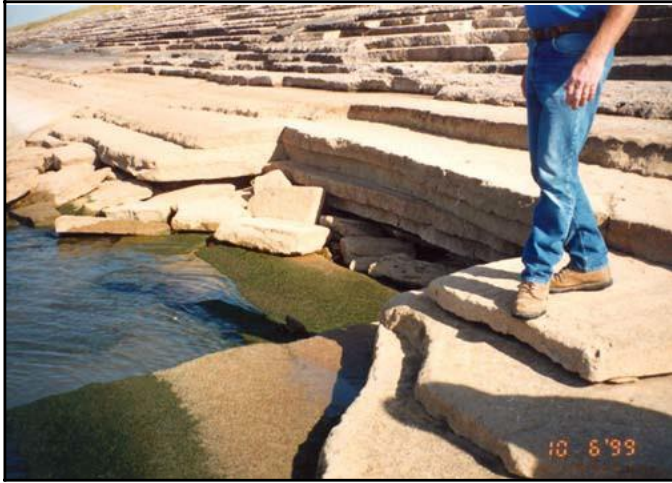
Figure 8-3. Upstream soil-cement slope protection showing damage from weakly bonded lift lines and freeze-thaw cycles.
