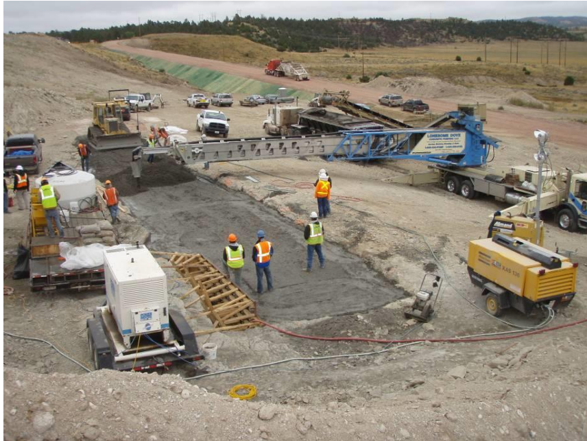
Figure 10-34. Placement of RCC test section using a Telebelt and dozer for placing and spreading.
