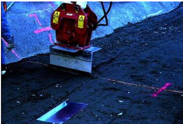
Figure 6-6. Galvanized steel sheet metal installation at Pueblo Dam to create a joint with a crack inducer.
