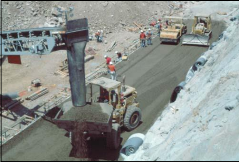
Figure 10-12. Delivery of RCC from conveyor belt to front-end loader on a lift at Camp Dyer Diversion Dam, with dozer and vibratory roller nearby.
