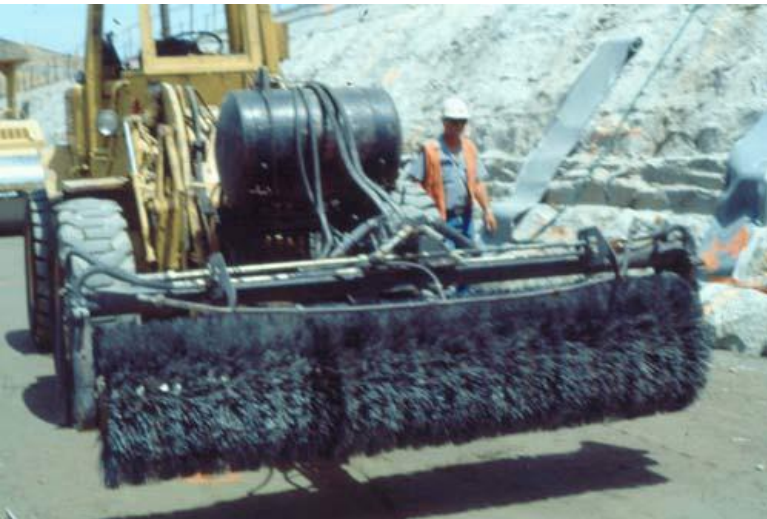
Figure 10-13. Power broom for cleaning RCC lift surface at Camp Dyer Diversion Dam.
