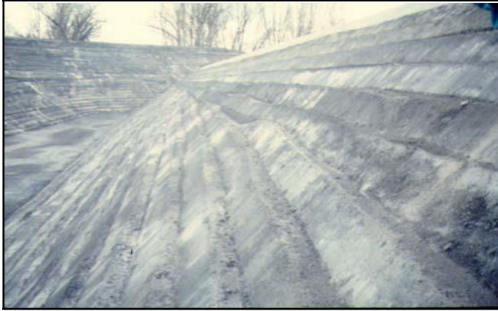
Figure 9-3. Stair-stepped slope downstream from the spillway crest.
