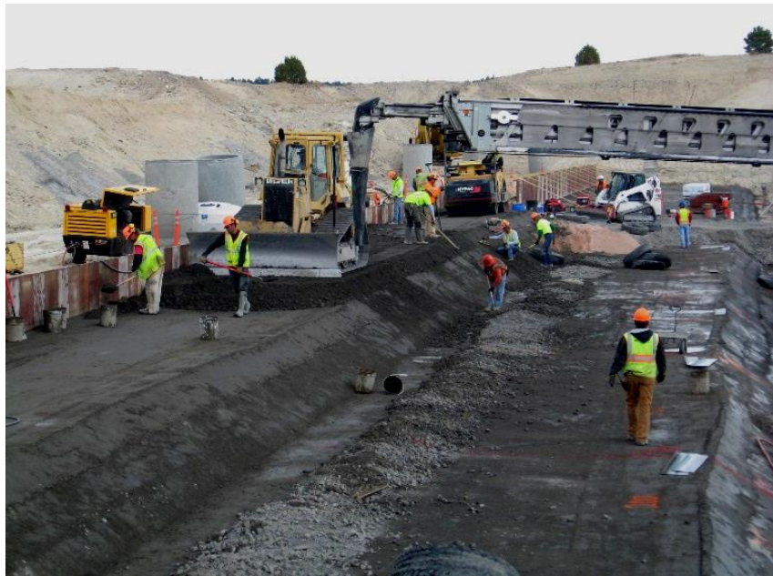
Figure 10-38. RCC placements in the upper portion of the RCC auxiliary spillway cutoff.
