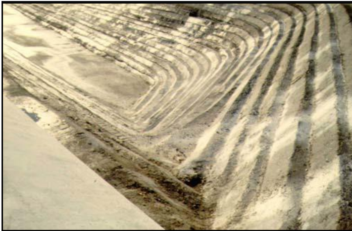
Figure 9-4. Tight radius corners at the upstream end of a spillway chute.
