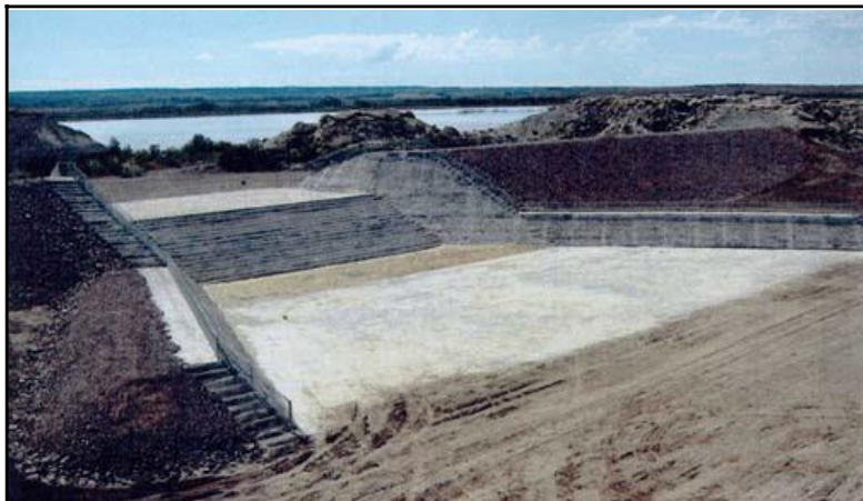
Figure 10-29. View of the completed spillway located in Dike BC of Many Farms Dam. Note the installed safety fencing and the sand backfill of the stilling basin.
