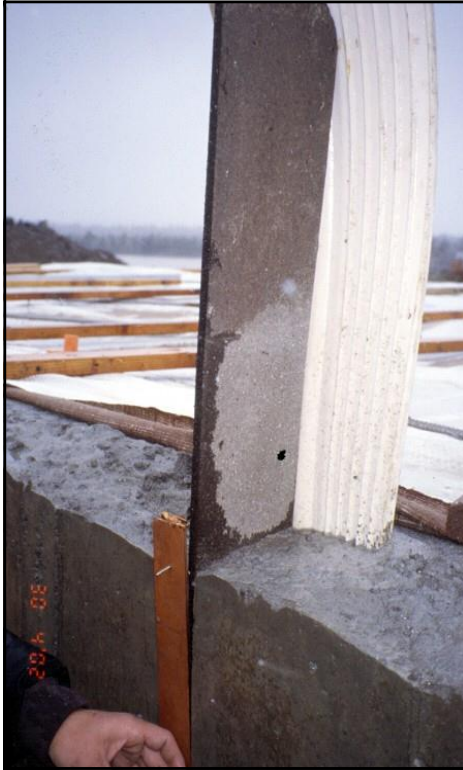
Figure 10-31. Contraction joint detail in formed upstream face of Clear Lake Dam, showing chamfer strip for sealant, ½-inch joint filler, and PVC waterstop within leveling concrete (from test section).
