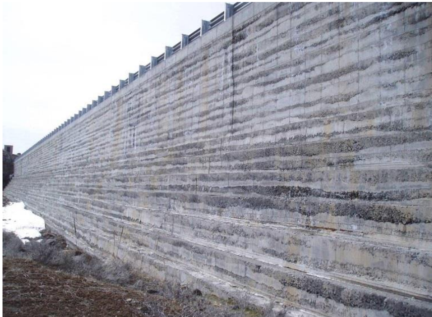
Figure 6-7. Photograph of the downstream face of Clear Lake Dam showing segregation that occurred against formwork.
