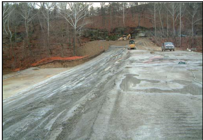
Figure 10-26. A view of Vesuvius Dam, Ohio, showing RCC armoring of the crest and downstream face.
