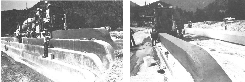
Figure 6-8. Construction of slip-formed facing elements at the test placement for Upper Stillwater Dam.
