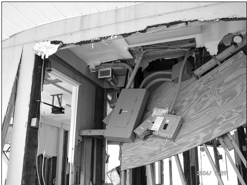
Figure 6. Non-compliant utilities attached to breakaway wall
