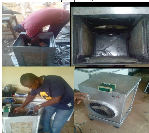
Plate 2.3d: Installation of suction fan, water grills, pump unit and humidity sensor
