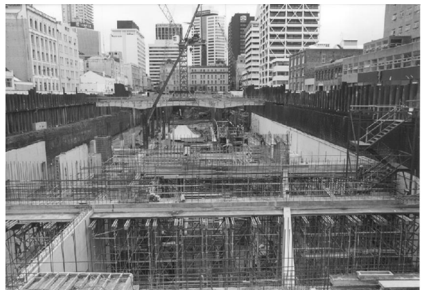
Photo 1 : View from East End. Bottom up construction in foreground with transition to Top Down frames in the distance.
