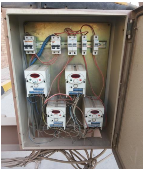
Fig. 18. Crane control unit
